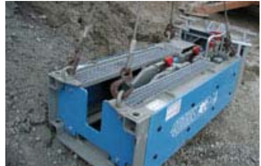
The NIBCO crew used a Grundoburst static bursting system like the one pictured here.
