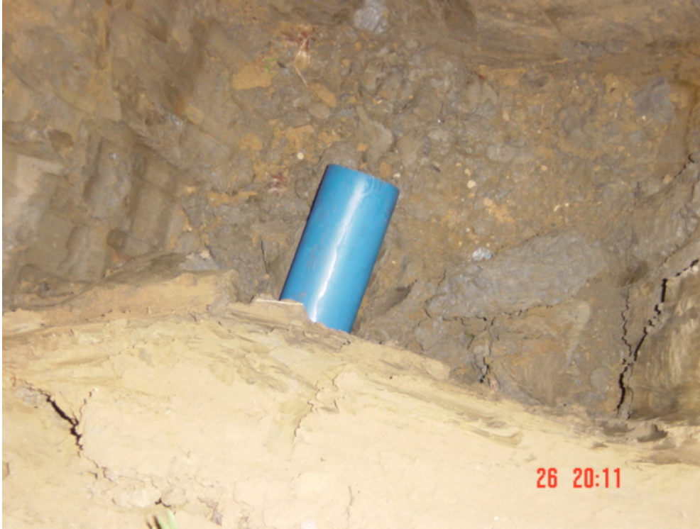
PHOTO 13 – Showing the 200mm \varnothing HDPE pipe for water connection was successfully installed.
