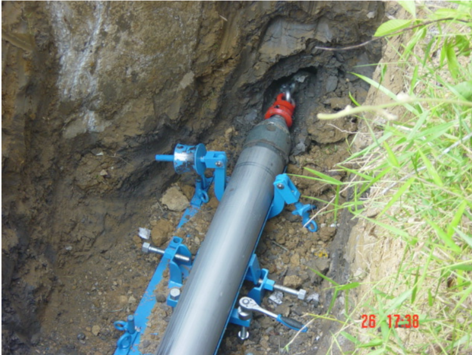
PHOTO 7 – The GRUNDOMAT 180mm \varnothing is reversed back to the starting pit with the winch cable.
