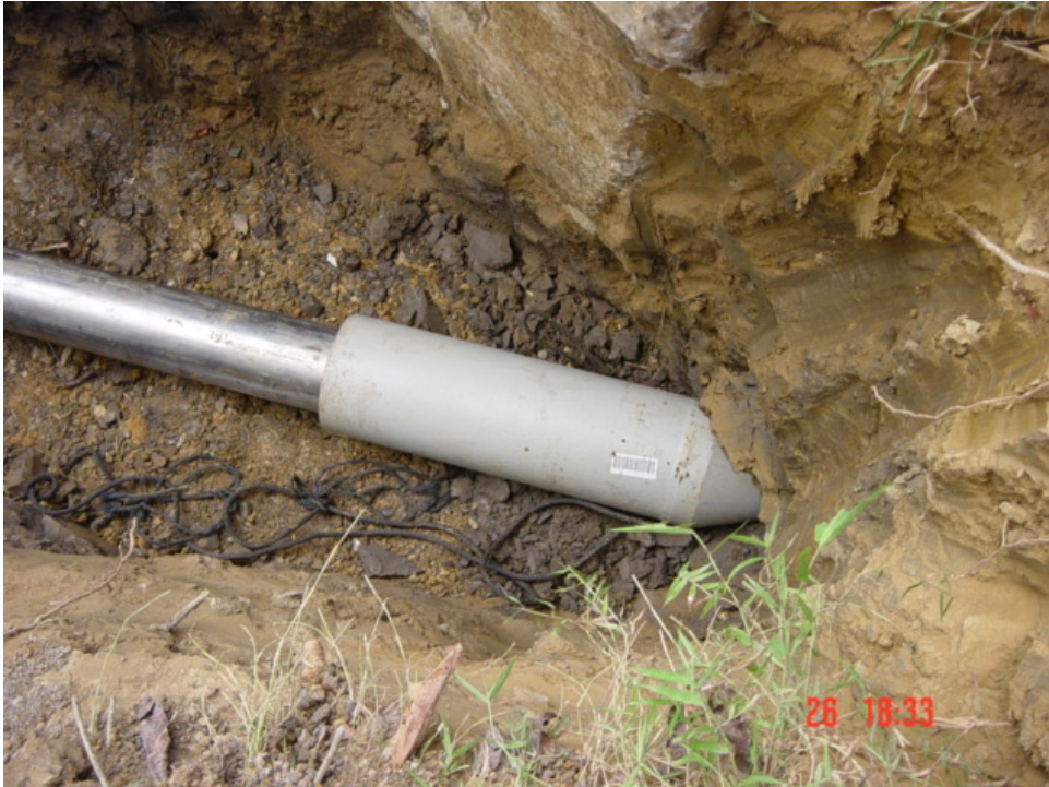
PHOTO 9 – Showing the the GRUNDOMAT with the Front-End Expander ready to bore through the existing borehole for upsizing.
