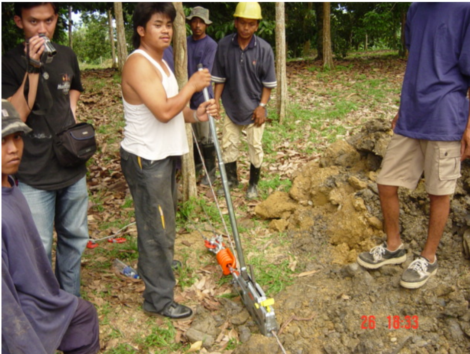
PHOTO 10 – Showing the the worker continue winching the 1.6t winch for tensioning at the reception trench.
