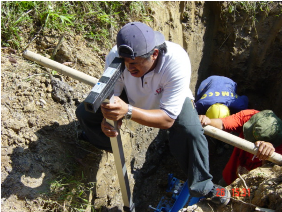
PHOTO 4 – GRUNDOMAT 180mm ø aligned in the starting pit ready for commencement of the 6m bore using Grundoscope.
