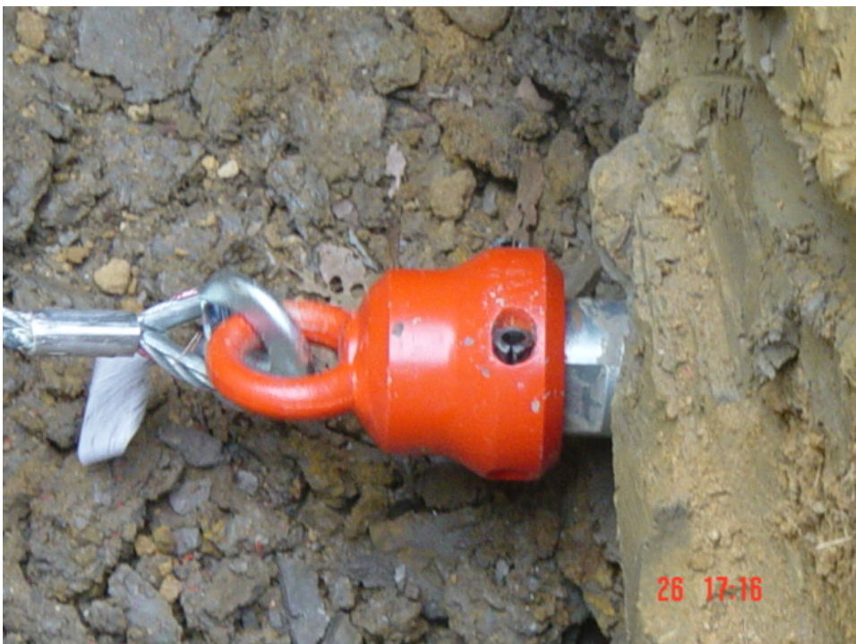
PHOTO 6 – A towing eye is attached to the GRUNDOMAT 180mm \varnothing to pull back the winch cable using the reverse mechanism of the GRUNDOMAT.
