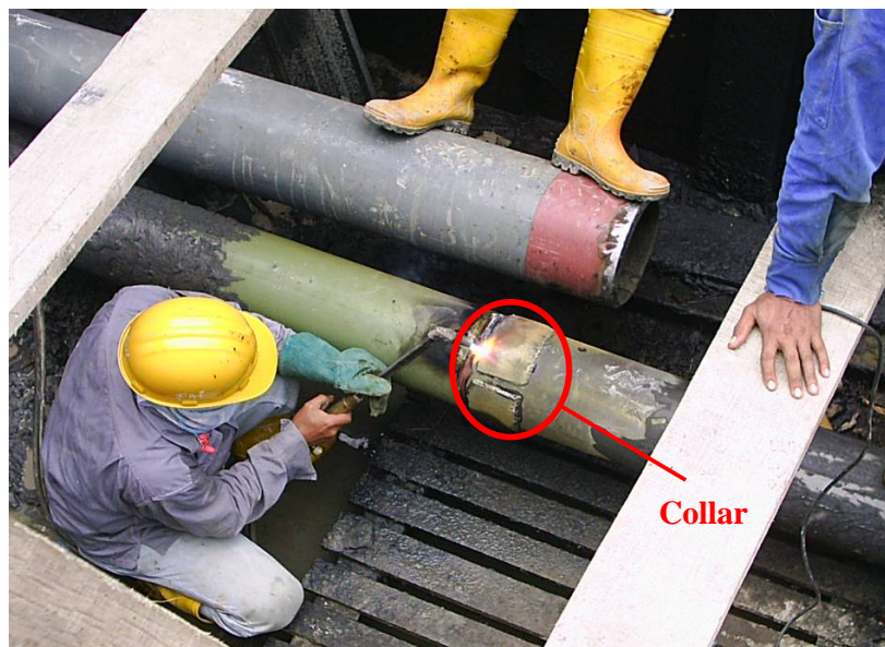
Photo 11: The new 8" Steel Pipe arrived at Pit B after 19 pipes were inserted. An improvised collar was welded onto the first pipe so as to act as a cutting shoe or prevent skin friction and also prevent the coating on the pipe being damaged.
