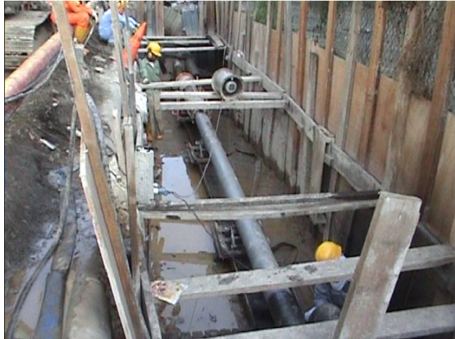
Photo 14: GRUNDORAM was being set up at Pit B for the ramming of 8" Steel Pipe to Pit C.
