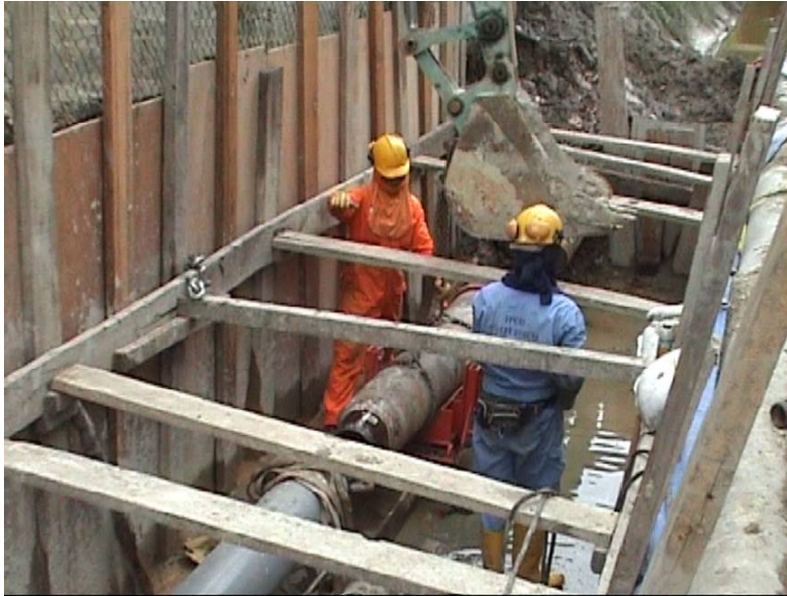
Photo 12: The GRUNDORAM was set up in Pit B for the ramming of the 10" Steel Pipe to Pit A.
