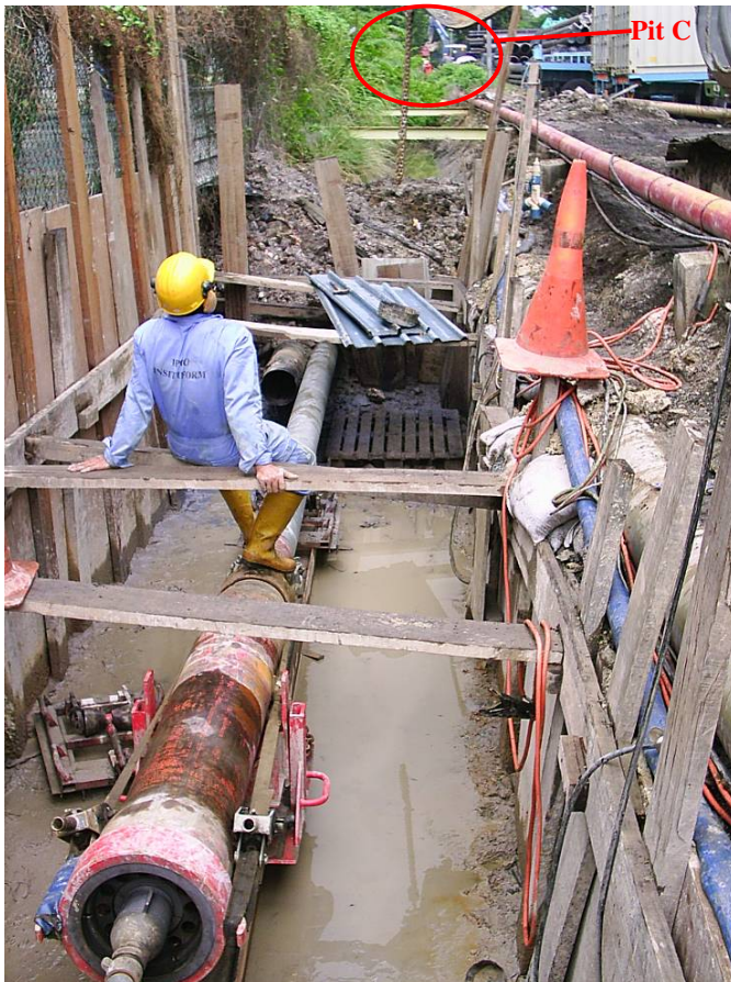
Photo 15: Another view of the GRUNDORAM in Pit B ramming the 8" Steel Pipe to Pit C.
