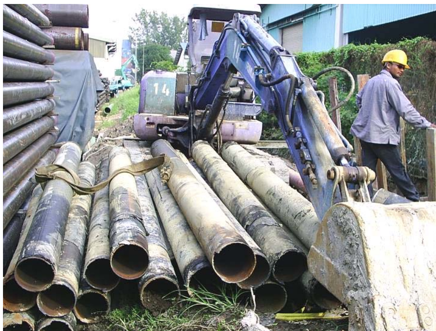
Photo 17: A view both the 8" and 10" old pipes that had been removed from Pit C.
