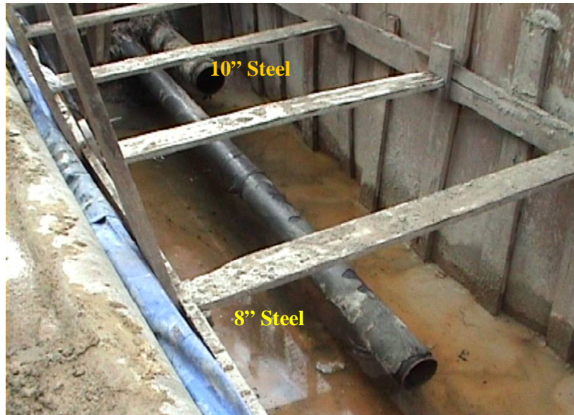
Photo 10: The old 8" Steel Pipe coming out at Pit B while the new pipe was being rammed in Pit A.
