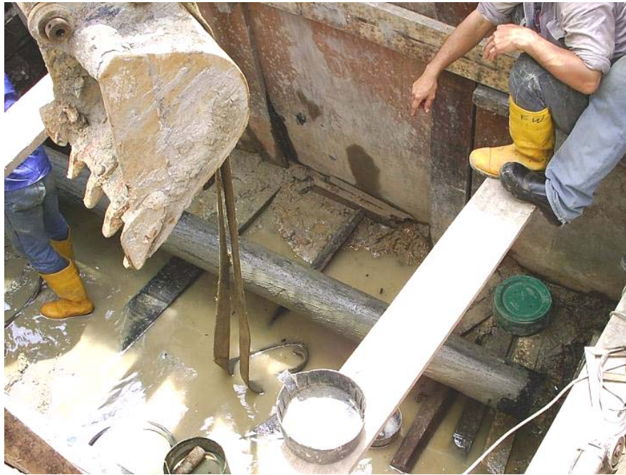
Photo 16: Arriving of the old 8" Steel Pipe at Pit C. Simultaneously, a new 8" pipe was welded in Pit B.
