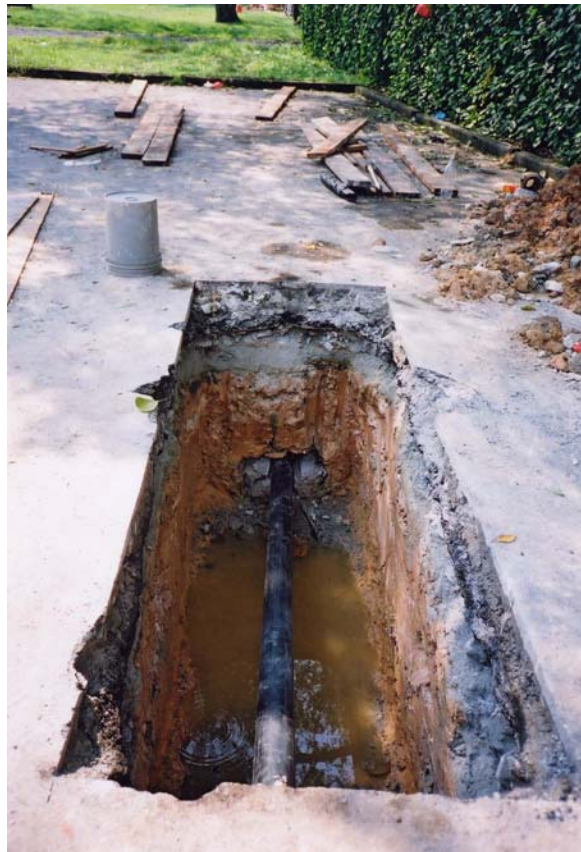
PHOTO 16 – View of 125mm PE pipe in the receive pit where a temporary connection to the existing sewer will be made until the next day's burst.
