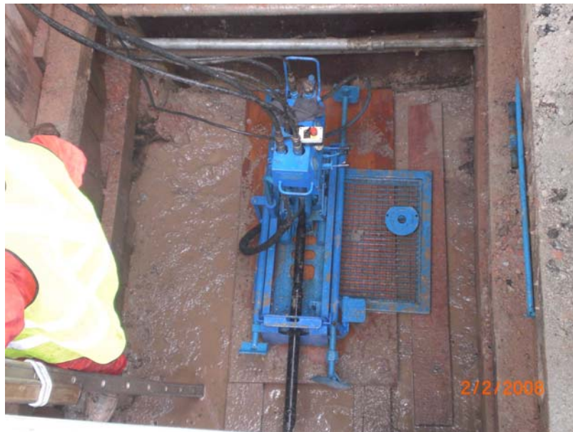
The entry/equipment pit was about 3 meters on width, 4 meters in length and 5 meters in depth. The reason to go so deep was to avoid the monsoon drain that was directly in front of the pit.
