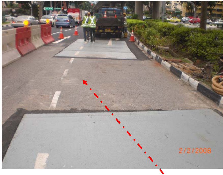
The objective of this job was to pull a Ø400mm HDPE pipe across the above drain culvert using trenchless method. Total length across the highway was about 14 meters.
