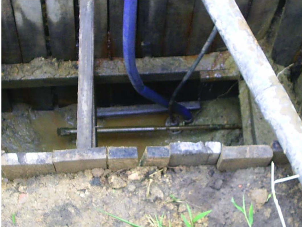
The drill head arriving on target at the exit pit. Total time taken was about 30mins.
